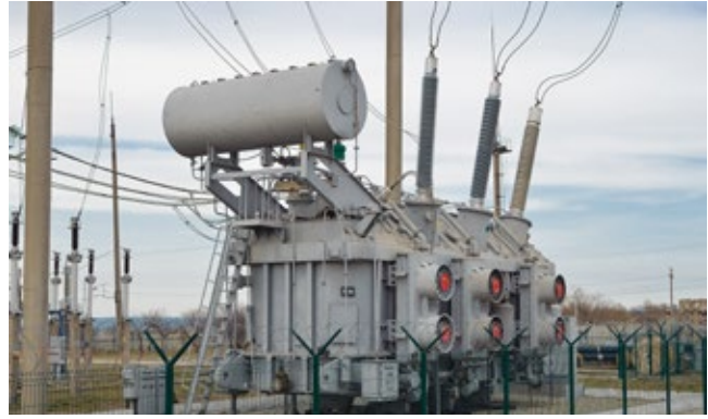
Transformer station: High energy demand makes megacities dependent and vulnerable Source: IABG
