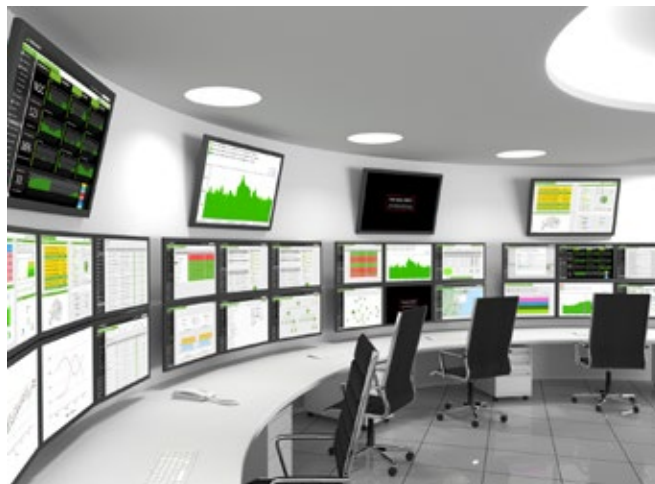
Network Operations Center: Artificial Intelligence will support real-time analysis and mission planning Source: IABG
